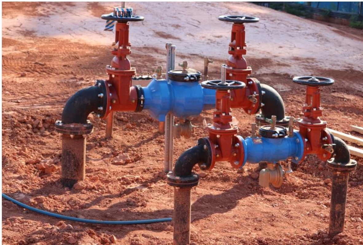
Backflow Prevention Assembly – East Side Near Mechanical Yard.
